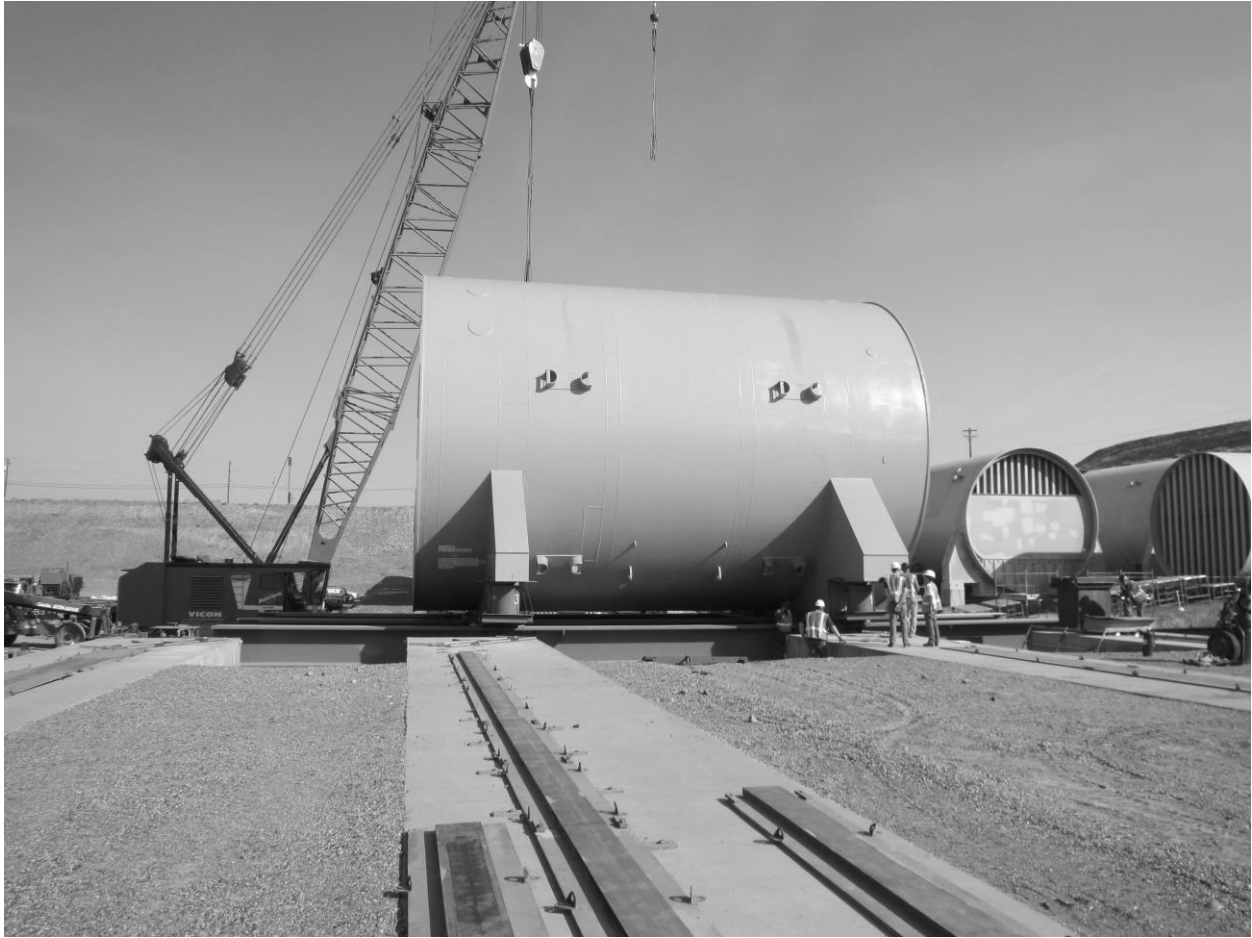
Preparing to move a Reactor Compartment Package into place on the Rail Delivery System in the Disposal Trench at Hanford
